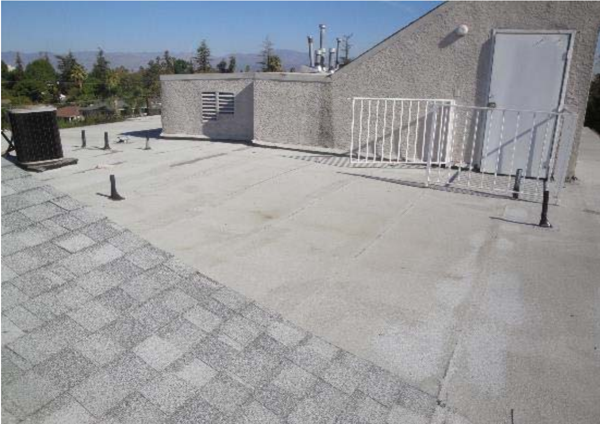
VIEW OF PROPOSED EQUIPMENT LOCATION
